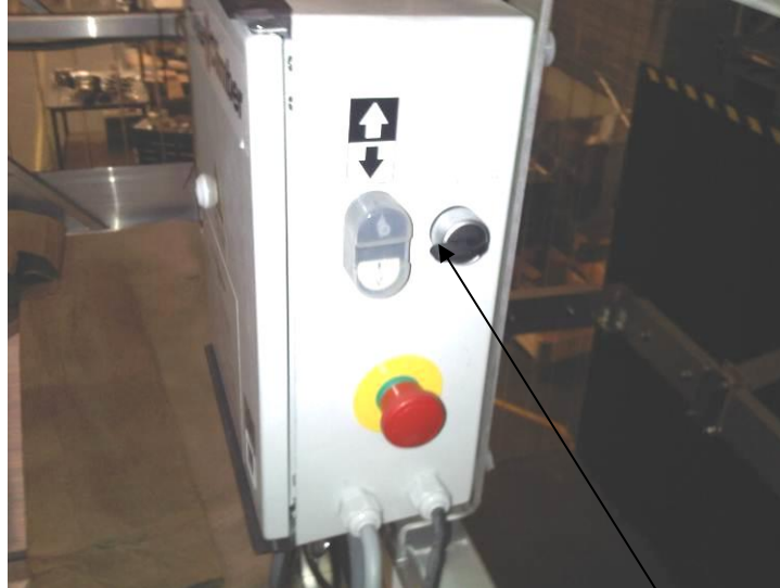
Pic 1 Selector switch for pendant control
