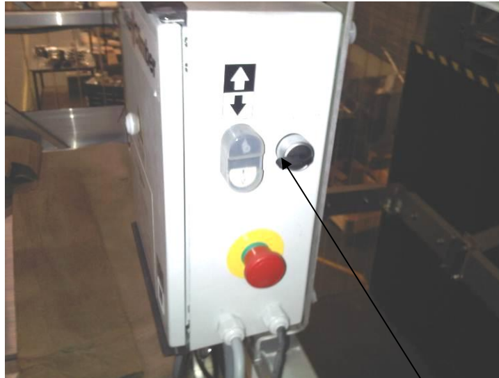
Pic 1 Selector switch for pendant control
